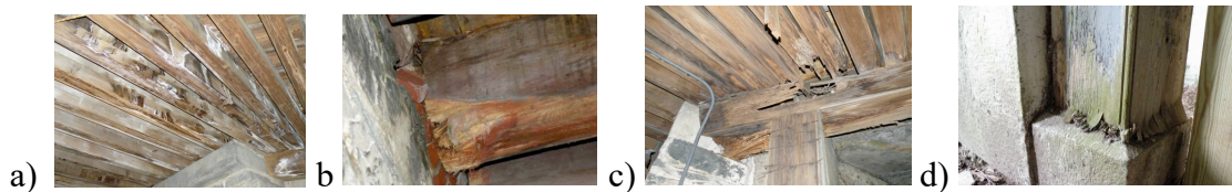
Fig. 8a,b,c,d. Moisture stains and efflorescence on joists within a corner casemate and arch; deteriorated girder and brooming at the base of a column.
